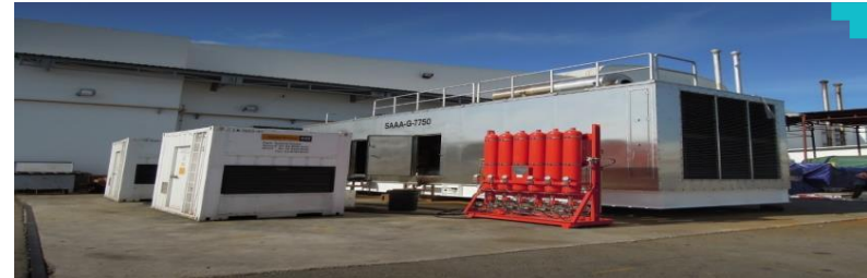
Diesel Generator Installed in SS316 Canopy, with Hydraulic Starting Skid
